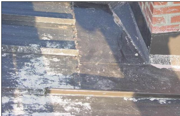
Figure 17-4 Mortar Droppings Should Be Cleaned Immediately.
