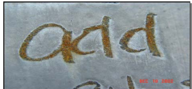
Figure 3 - 16 Roof Corrosion from the Use Of a Graphite Pencil
