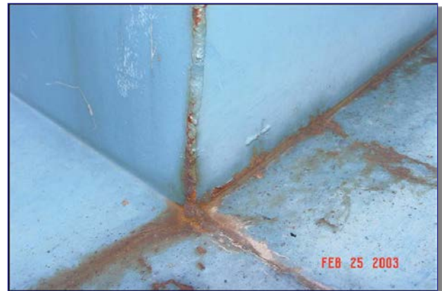
Figure 3-5 Corrosion Due To Welding - Coated Material Destroyed By Heat from Weld
