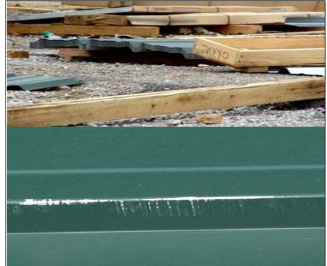
Figure 9-12 Improper Staging of Material Will Cause Damage
