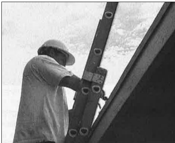
Figure 9-5 Extend the Ladder At Least 3 Feet Above the Eave and Tie It Off
