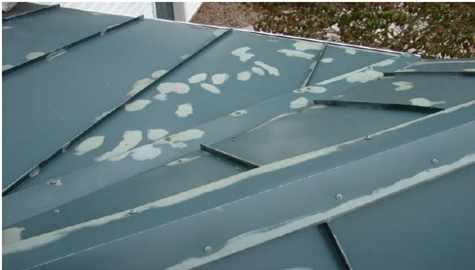
Figure 1 - Appearance of a pre-coated metal roofing where a low performance field applied air-dry paint system was used
