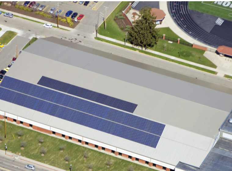
The Peterson Field House at the University of Mount Union (Alliance, Ohio) generates its own electricity, thanks to the installation of a 6132-m 2 (66,000-sf) PV roof system that ranks as the largest single solar array, thin-film laminate system in Ohio.
