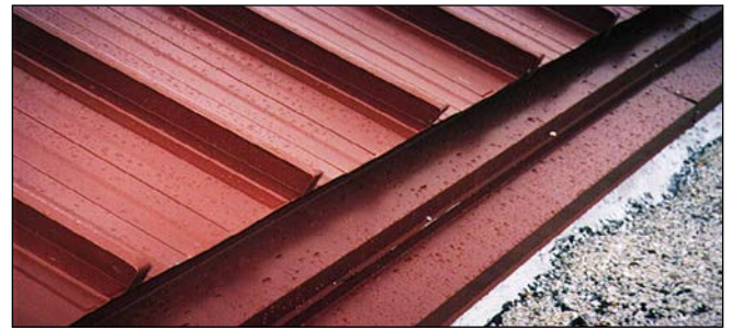
Figure 4-19 Hydrokinetic Roofs Are Designed to Deal with Moving Water, Often in Large Volumes
