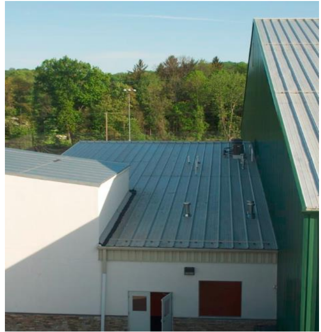
Figure 4: Some building and roof geometries can create “drift loads”
