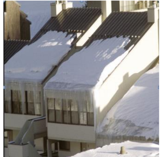
Figure 6B: Ice dams create unintentional snow retention
