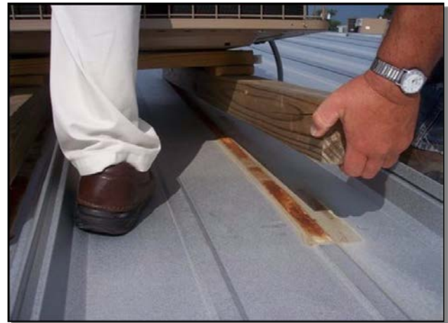
Figure 3-15 Roof Corrosion from Treated Wood
